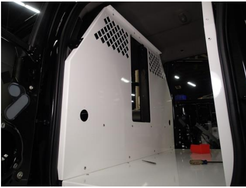
Attach front wall to "B" pillar brackets and floor using 1/4" x 3/4" carriage bolts and serrated nuts.
