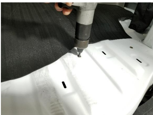
Install 1/4" rivnuts into the holes and tighten using a rivnut gun or rivnut tool.
