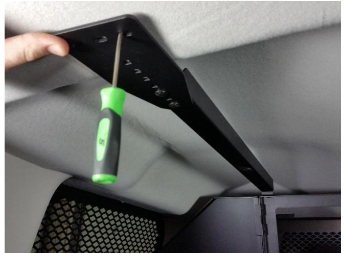
Verify sheet metal above headliner once bracket is lined up using a straight pick tool.
