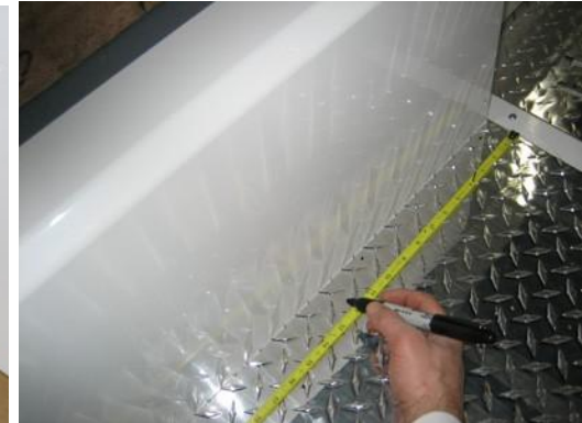
Attaching Floor Measure every 9.5" inches or approximately 7 diamonds and make a mark for the floor screws.
